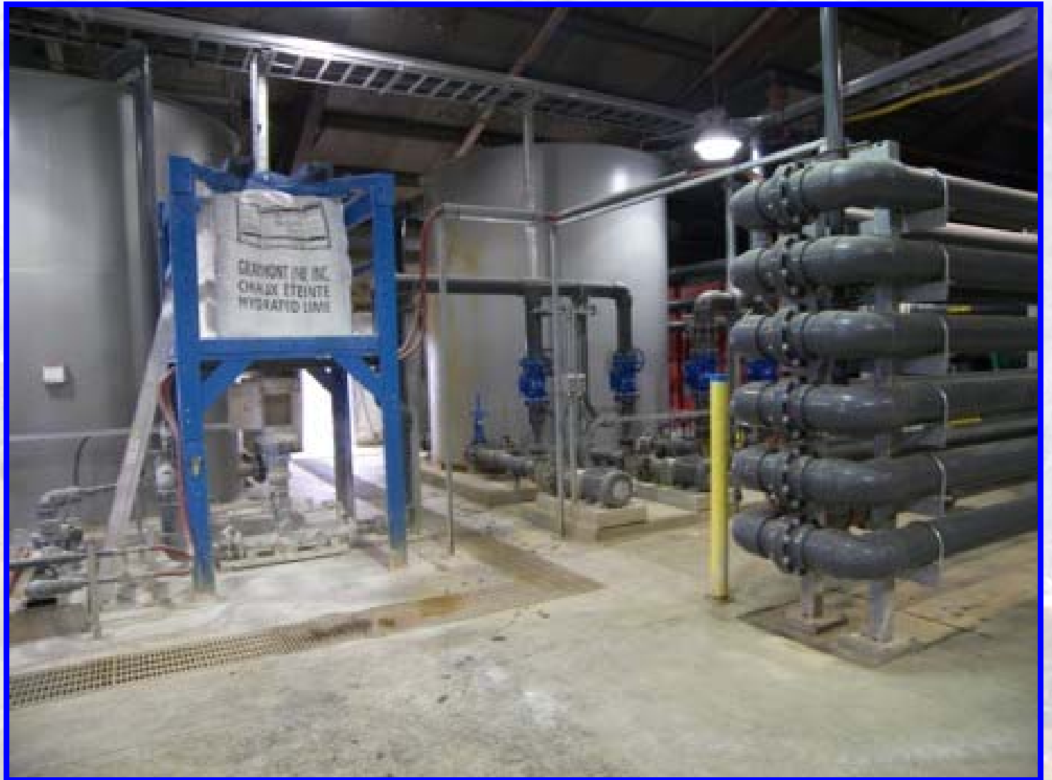
Waste water treatment plant at the Ming Mine site
