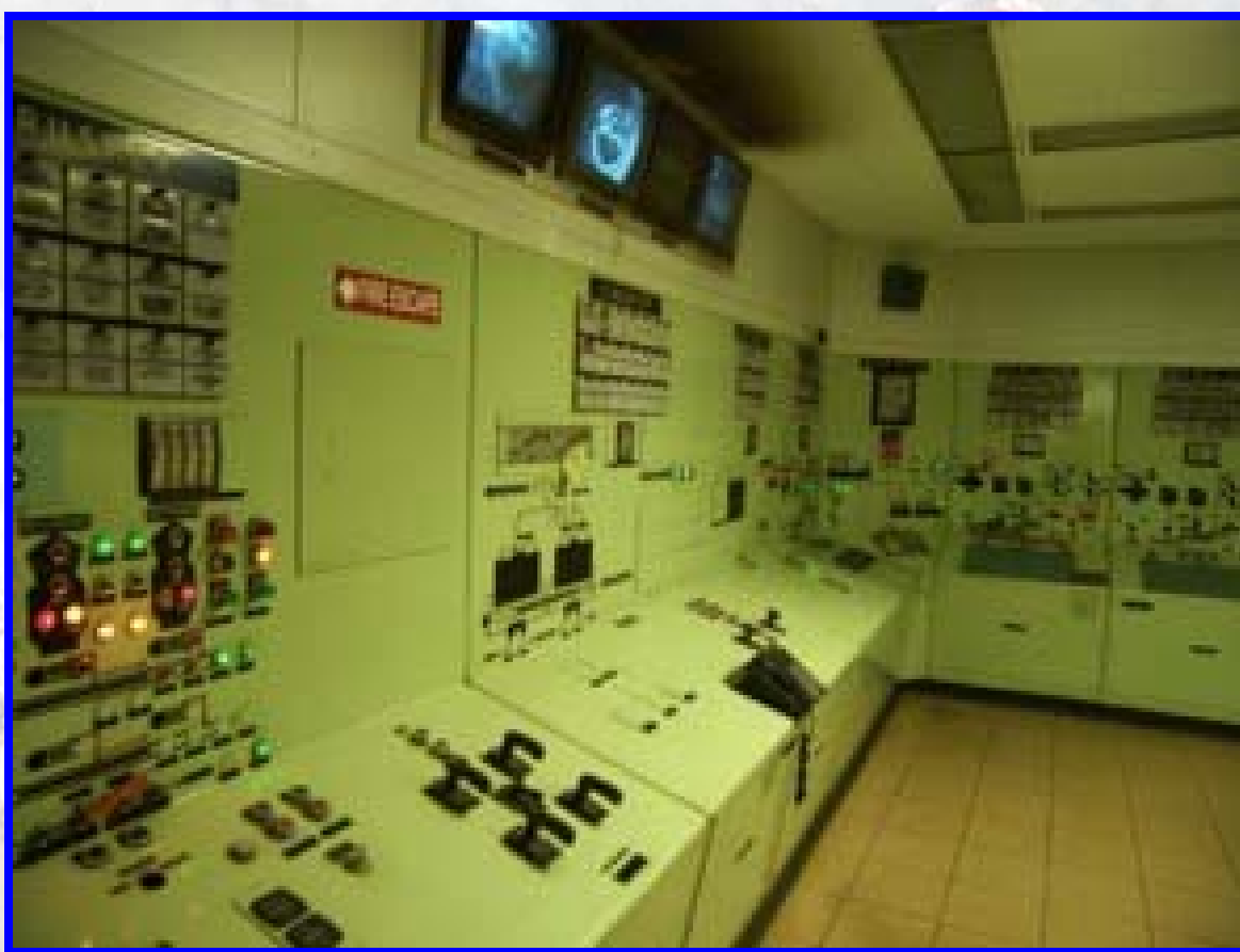
Mill control room – Wabush Mines
