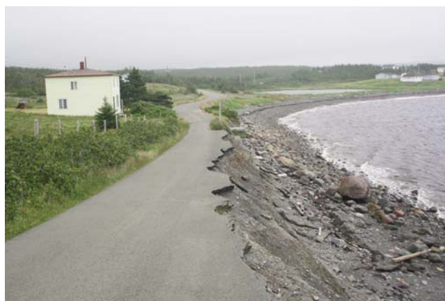
Plate 3. Coastal erosion at Admiral's Beach, Avalon Peninsula, undercut this transportation route.
